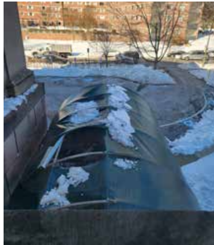
Heavy snow and ice sliding off of the temple roof caused significant damage to the awning of the 39th Street Entrance
